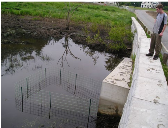
Figure 9. Flow device constructed of stout fencing material used to prevent beavers from blocking the movement of water through a road culvert. (Photo, “ Trapezoidal Culvert Protective Fence Westford, MA ” by Michael Callahan, 2004, https://commons.wikimedia.org/w/index.php?curid=9449818 and licensed under CC BY-SA 3.0 , https://creativecommons.org/licenses/by-sa/3.0/?ref=openverse .)
